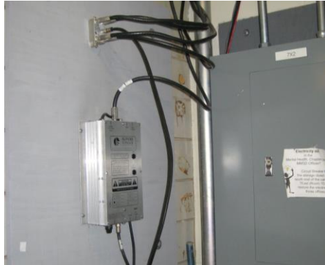
Photo 4: Seventh Floor CATV Distribution
