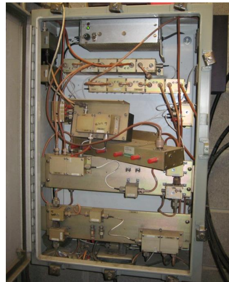
Photo 19: RF Distribution Equipment
