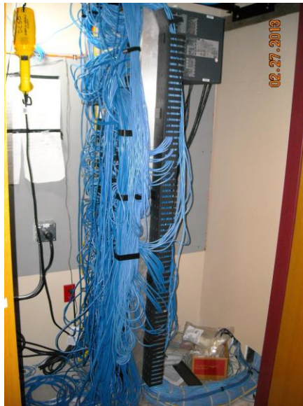
Photo 14: Second Floor Telecommunications Room
