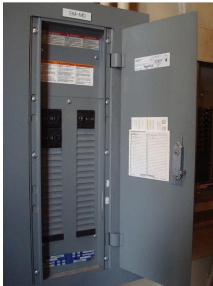
Panel EM-DP (Sixth Floor East Electrical Room)
