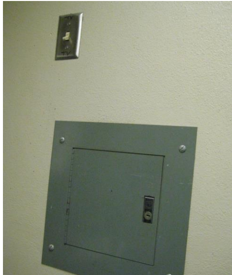
Photo 5: CATV Cutoff Switch
