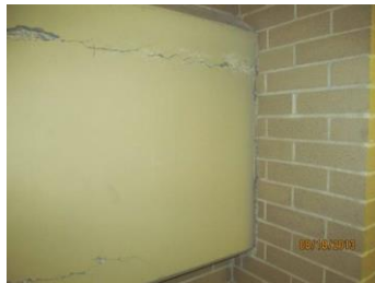
Photo 14: Stairwell structural damage
