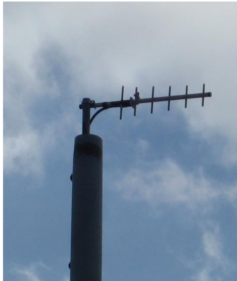
Photo 9: Exterior Yagi Antenna
