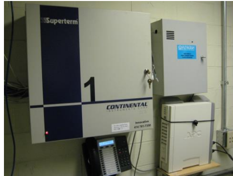
Photo 6: Access Control System
