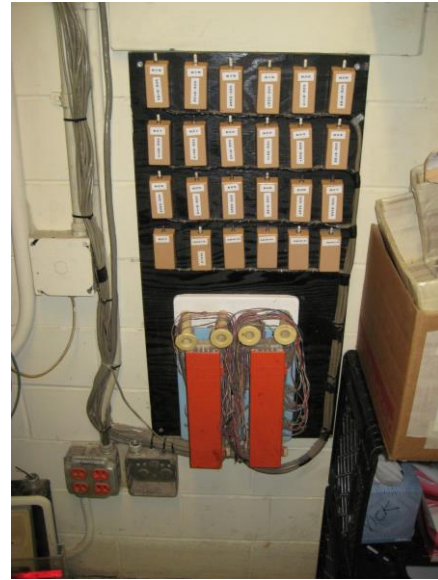
Photo 3: Inmate Telephone Cutoff Switches
