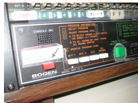
Photo 83: Second Floor Intercom System
