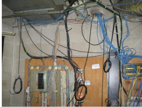
Photo 2: Voice/Data Horizontal Cabling
