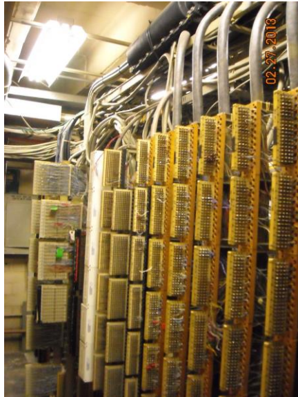
Photo 1: MDF (Main Distribution Frame)
