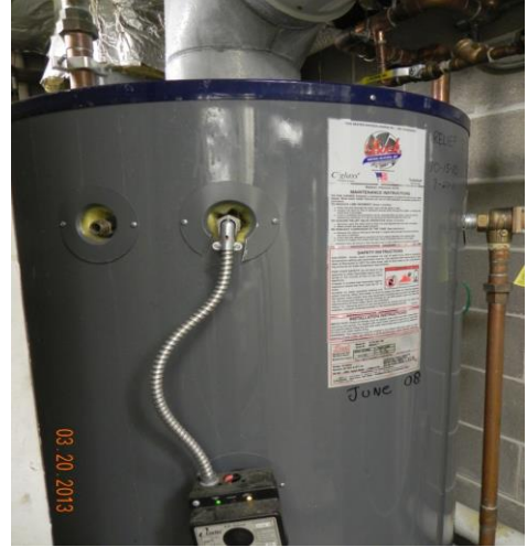
Second Floor Domestic Water Heater
