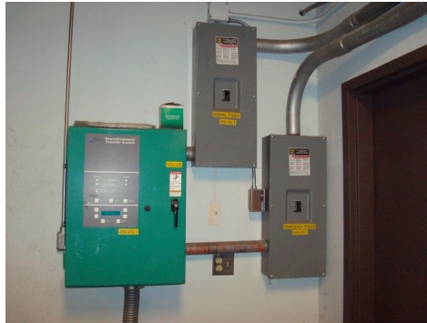
125A Enclosed Circuit Breakers and ATS #2E (North Wall Generator Room)
