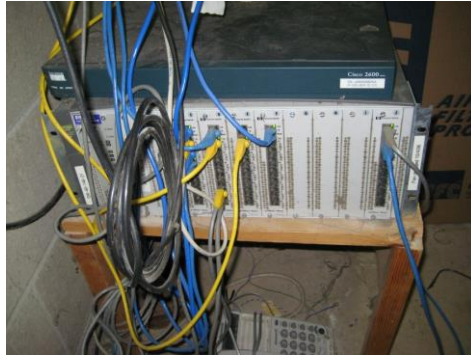
Photo 3: First Floor Network Switch
