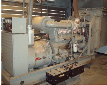
260 kW Packaged Generator Set (Penthouse Generator Room)
