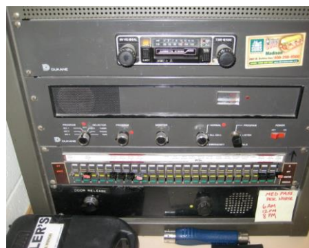
Photo 72: First Floor Intercom System
