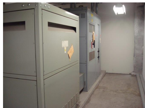
MDP-2P and 750 kVA Transformer (Penthouse Electrical Room)
