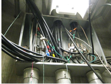
Photo 19: RF Distribution Cabling
