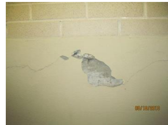
Photo 15: Stairwell structural damage
