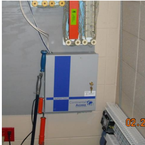
Photo 15: Non-secure Access Control System
