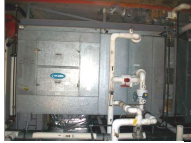
Air Handling Unit in Penthouse
