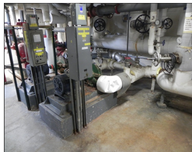
Existing East Building Domestic Water Booster Pump (Original to Building)
