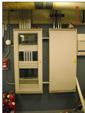
Building FACP (Ground Floor)
