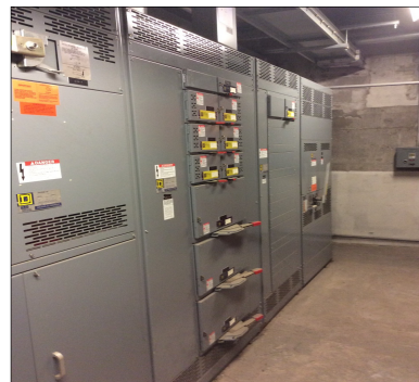
3000A, 208Y/120V West Switchboard (Ground Floor Electrical Room)
