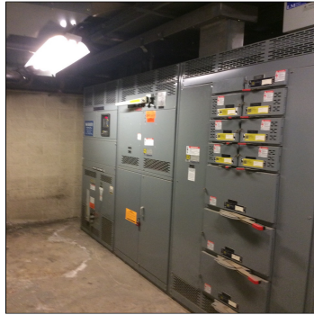
300A, 208Y/120V East Switchboard (Ground Floor Electrical Room)
