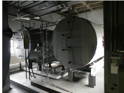
Existing 3500 Gallon/Ea. Domestic Water Storage Tanks East Penthouse
