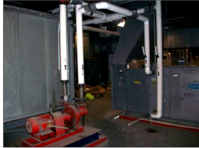
Air Handling Unit and Heat Recovery Pump
