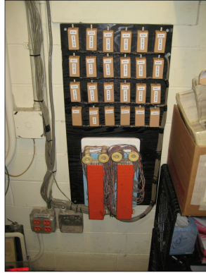
Inmate telephone cutoff switches
