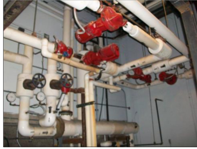
Steam to Hot Water Converter and Pumps
