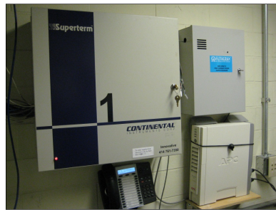
Access Control System
