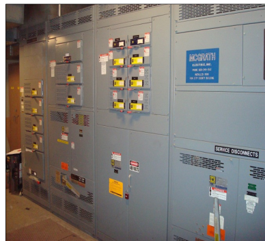
400A, 480Y/277V Switchboard (Ground Floor Electrical Room)
