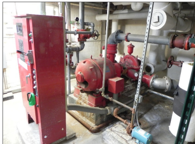
Existing Fire Pump and Jockey Pump East Building
