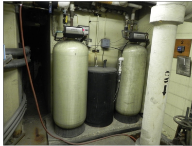
Existing West Expansion Water Softeners (Original to Expansion)
