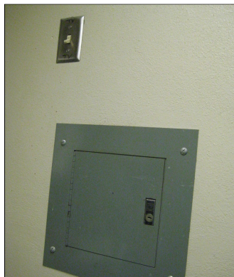
CATV Cutoff Switch
