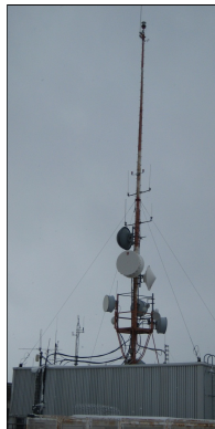
East Roof Antenna
