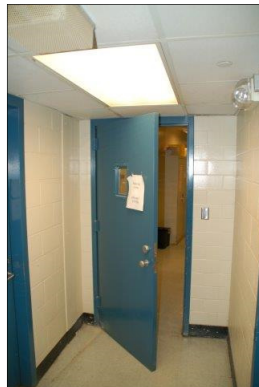
Door at Smoke Barrier
