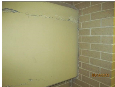
Stairwell Structural Damage
