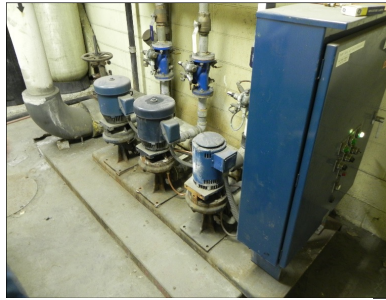
Existing West Vertical Expansion Domestic Water Booster Pump System
