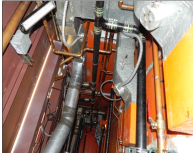
Cell Chase Showing Uninsulated Domestic Water Piping. Code Requires Domestic Water Piping to be insulated.
